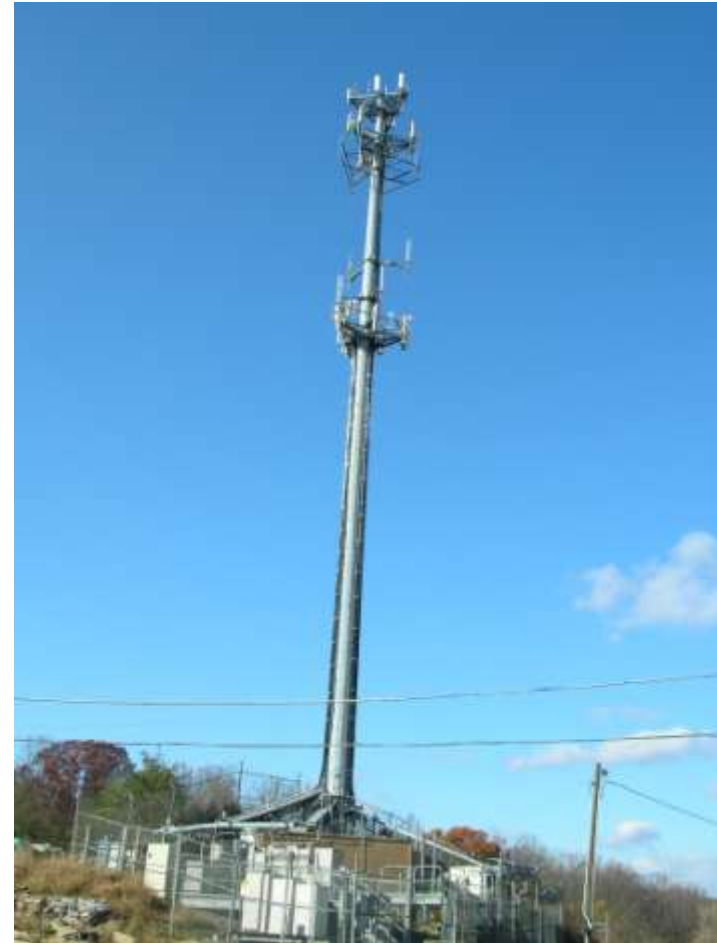
Monopole with Equipment
