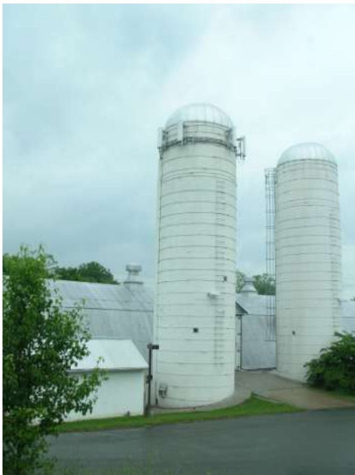
Antennas Mounted on Silos
